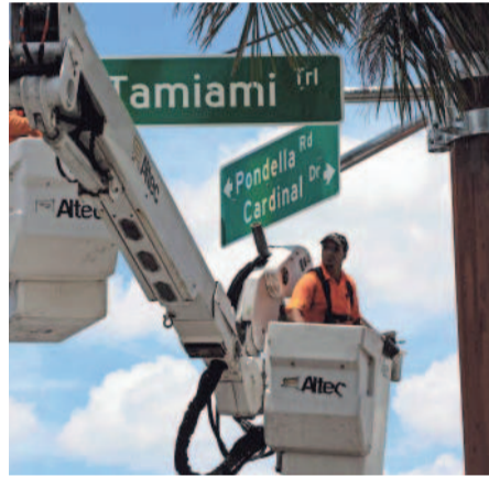
Lee County Department of Transportation signal technicians install road signs on Friday 2019, at the intersection of Pondella Road and US 41 in North Fort Myers. JON AUSTRIA/NAPLES DAILY NEWS USA TODAY NETWORK - FLORIDA
